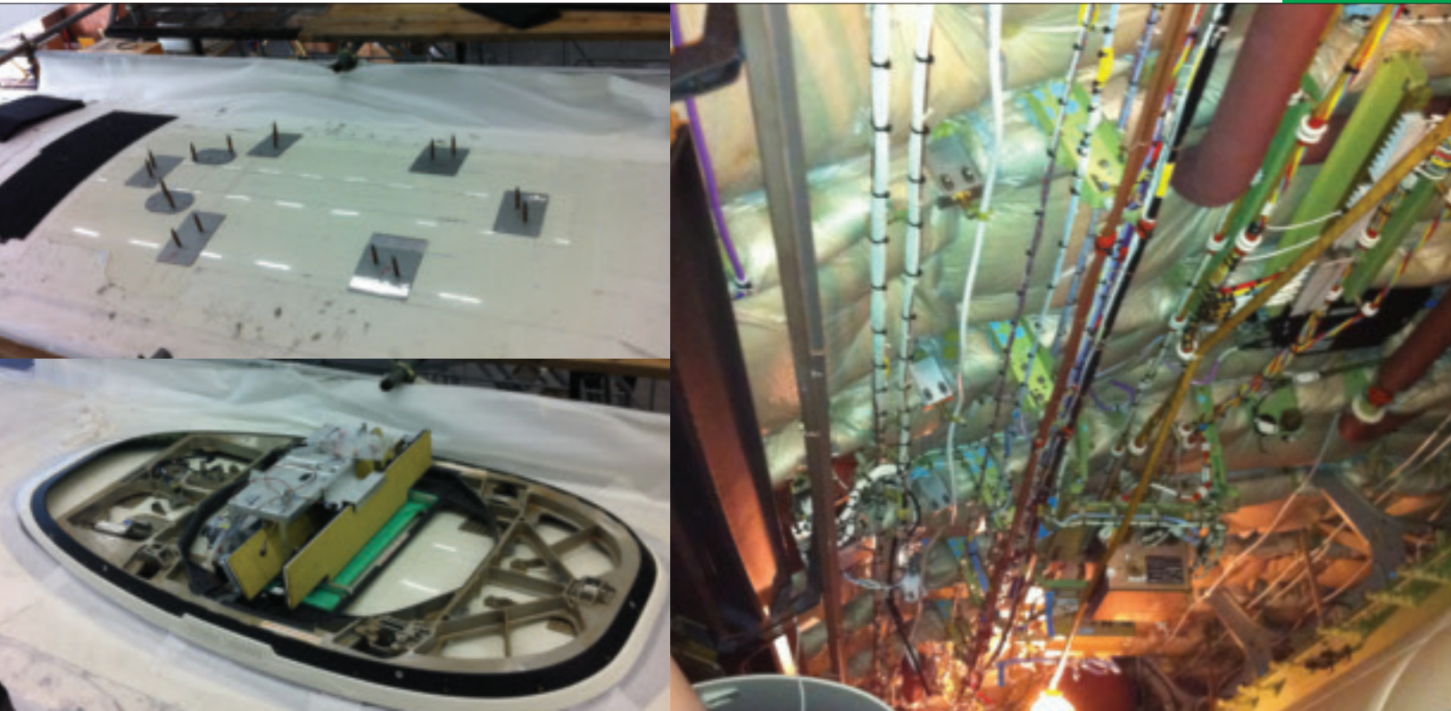
From left: Engineers from Turkish Technic were involved throughout the STC process; Centre: After the installation of external fittings and doublers, the adapter plate and the adapter plate skirt installed. After the application of required preventive compounds the antenna installed on the adapter plate. Right: Leaky feeder cables and data cables were installed for the GSM system through the cabin.
