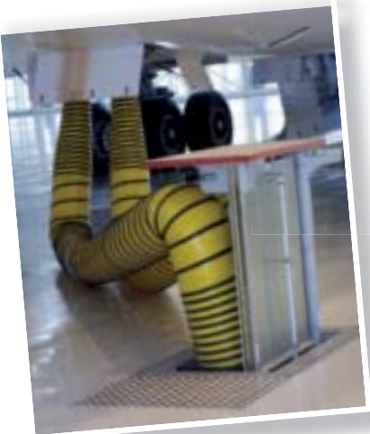
Cavotec's pop-up units deliver a full range of utility services – from air and water, to fuel and power – and retract back into the tarmac when not in use.
